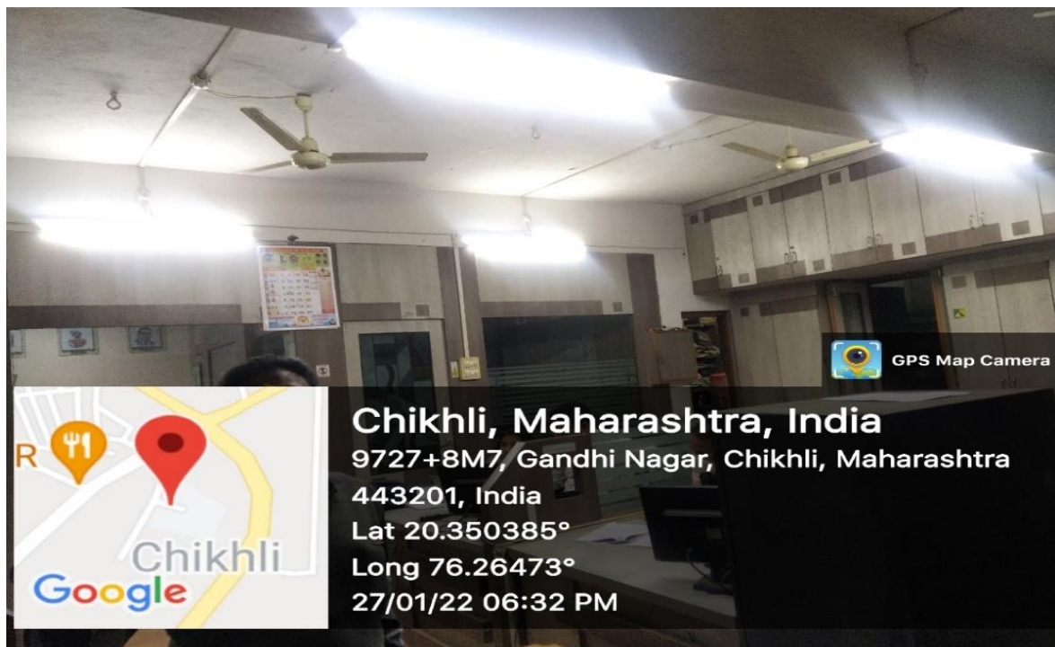
LED Tube Lights: Administrative Office
