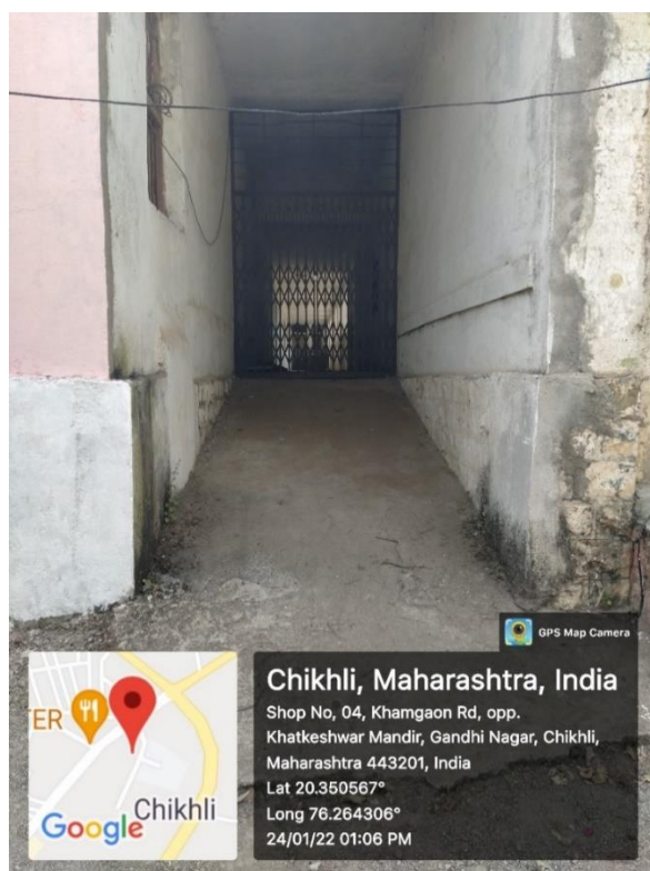
Divyangjan-Friendly, Barrier Free Environment: Ramp-5 For Classrooms
