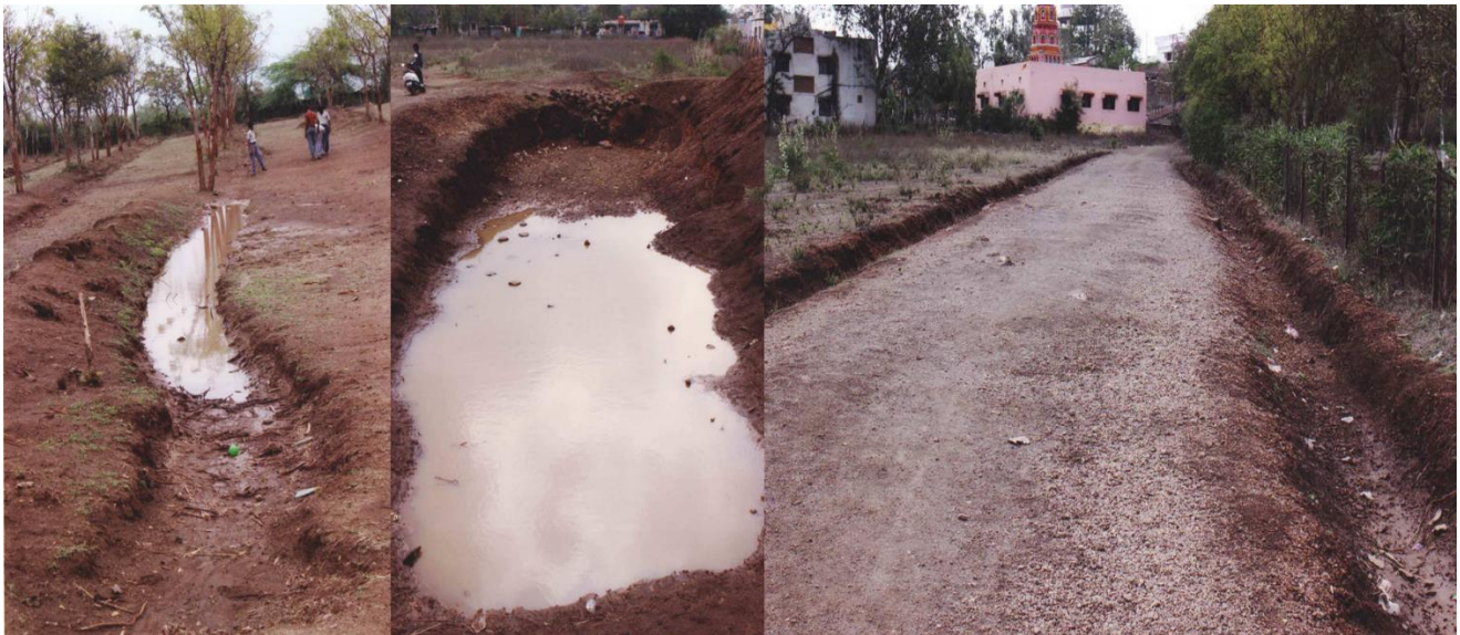
Recharge Trenches for Precipitation of Rain Water
